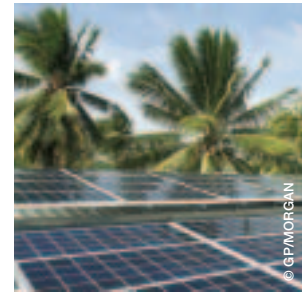
image Solar panels on refrigeration plant (for keeping fish fresh), Likiep Atoll, Marshall Islands.
