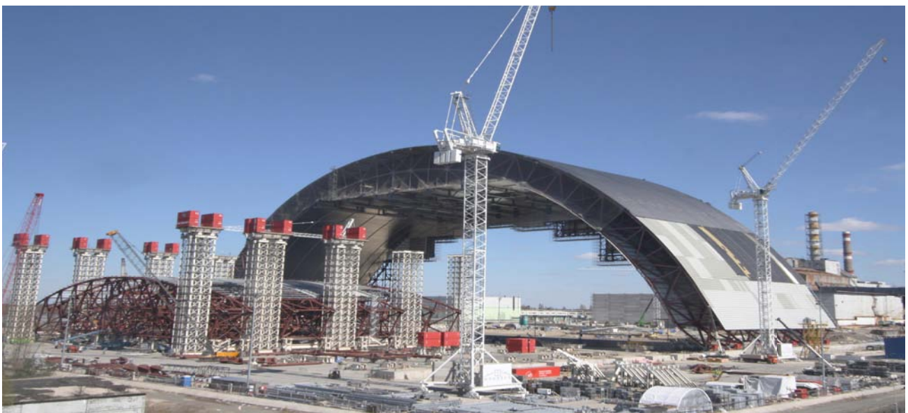
Fig. 41 Assembly of second bay structure. On background the first displaced structure (source chnpp.gov.ua)
