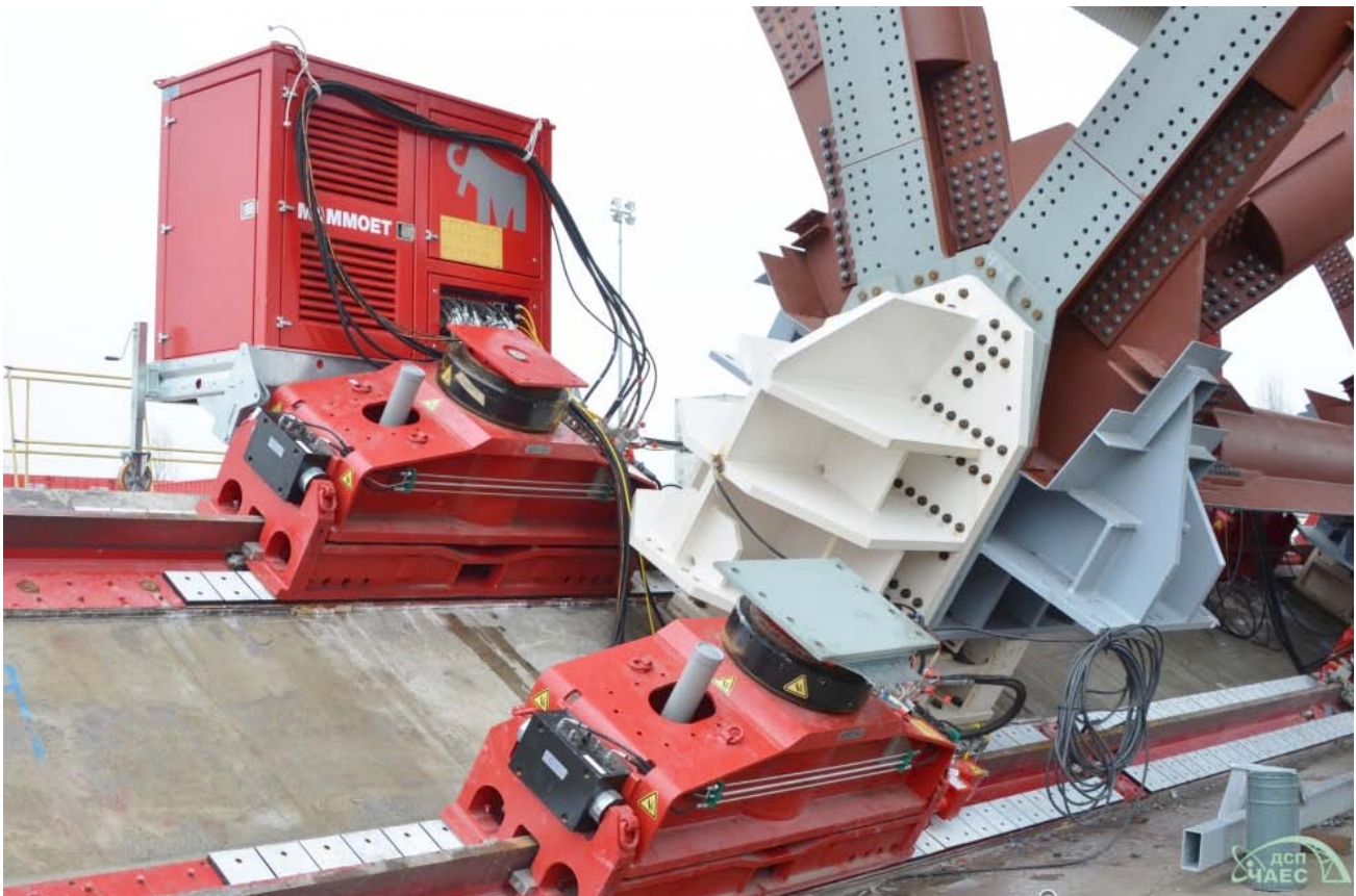
Fig. 44 Details of rolling structures to slide the NSC to final position (source chnpp.gov.ua)
