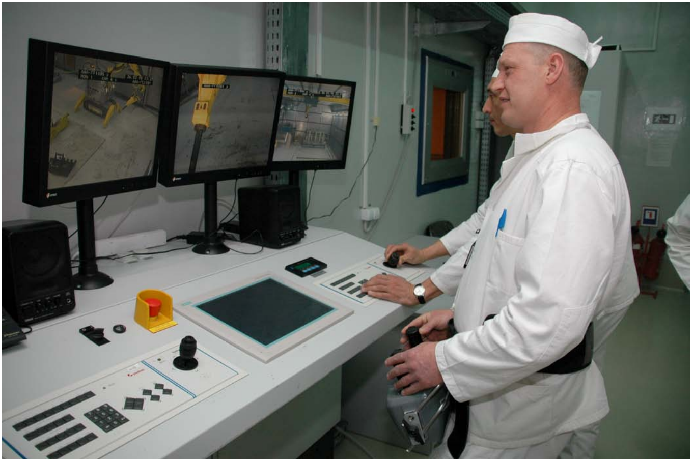
Fig. 34 ICSRWM – Control Room (source chnpp.gov.ua)
